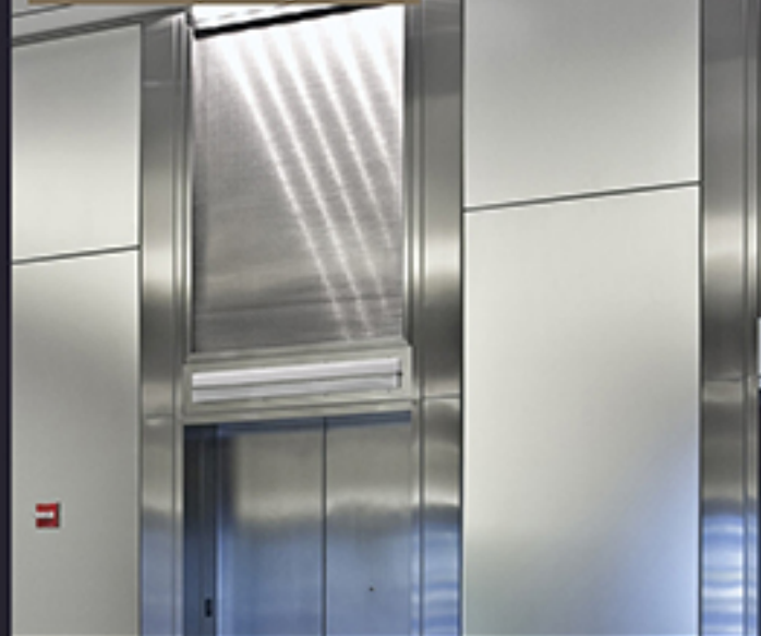
Elevators/ Cargo Lifts
